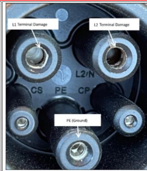
Figure 2: Charger Gun Terminal Damage
