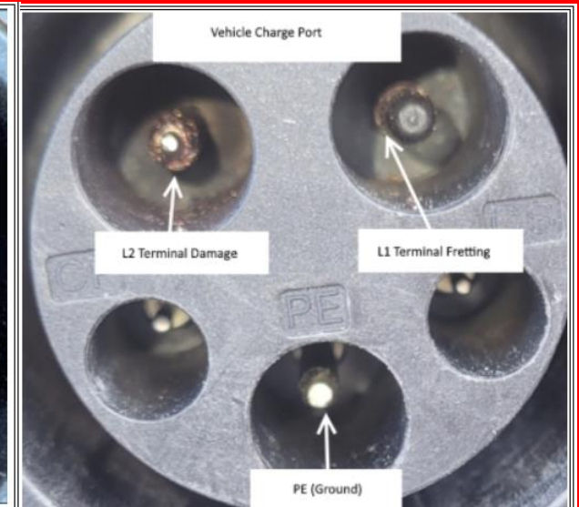
Figure 3: EV Vehicle Charge Port Damage
